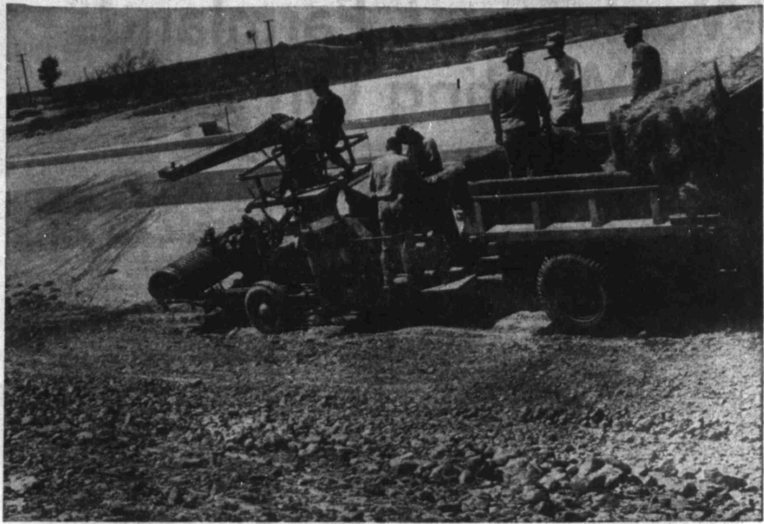
HIGHWAY DEPARTMENT USES BIG GUN IN ITS MODERN WAR ON EROSION Pulverized hay, blended with asphalt, employed in grassing IS 20 bypass embankments
