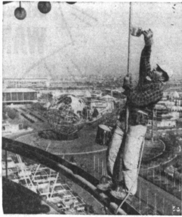
SUPPORTING ROLE — Worker is on precarious perch in painting supporting cable on New York State Pavilion of New York World's Fair. Unisphere is in background.
