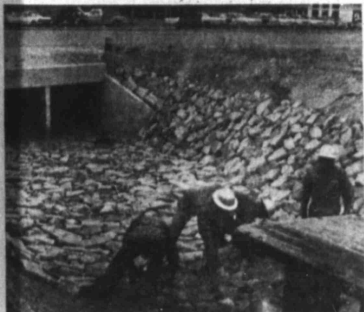
DRAINAGE PROJECT NEARS COMPLETION New 600-foot drainage area on East Fourth Street
