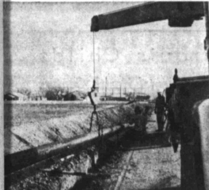
WATER LINE GOES IN FOR CEMETERY As part of improvements under new permanent care plan
