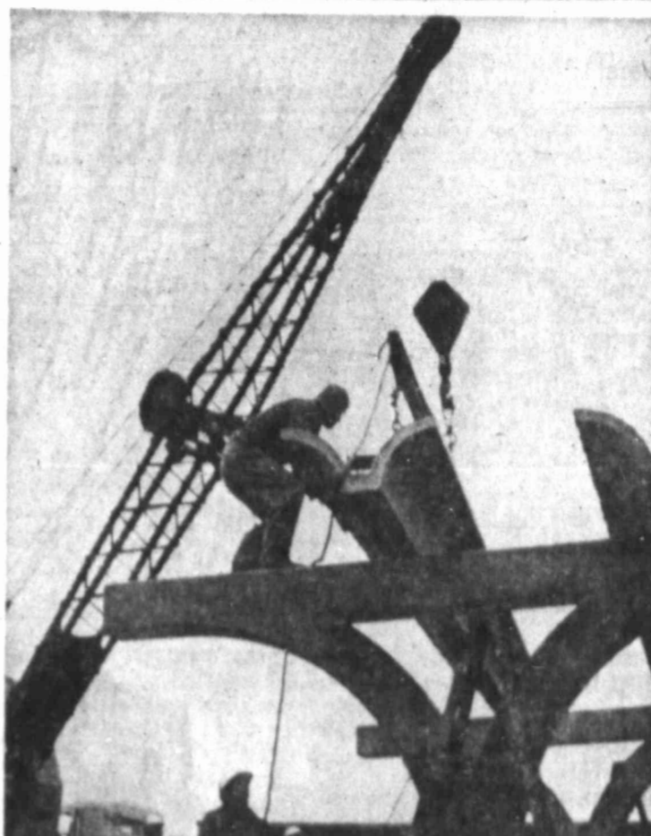
COMPLETE MOSS CREEK LAKE ADDITION Roof goes on the second picnic pavilion
