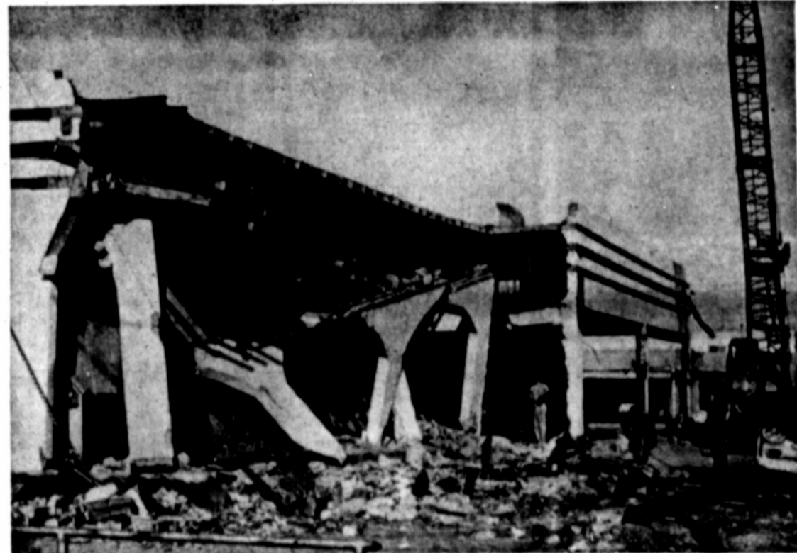
WRECKERS BATTER DOWN OLD ICE PLANT WALLS structure to be remodeled into spaces for five stores
