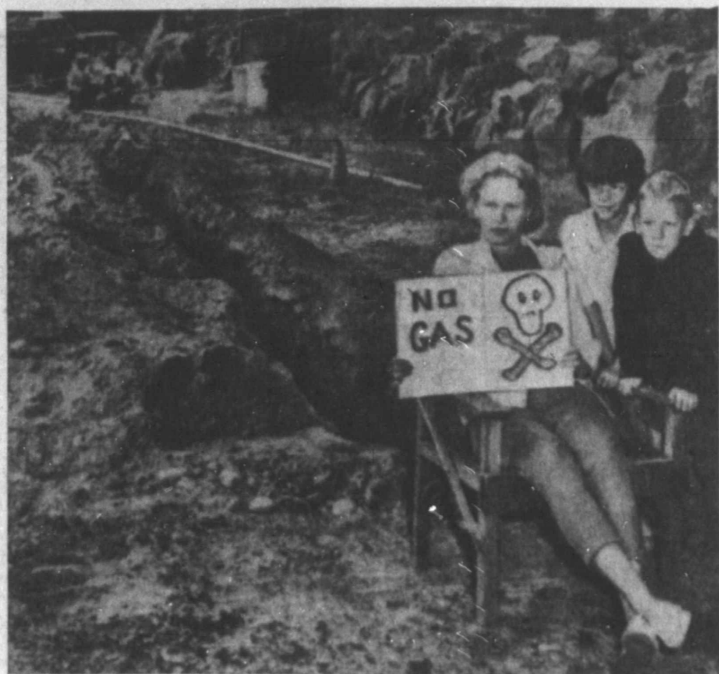
Pipeline Impasse Mrs. Marjorie White, 29, Seattle housewife, is staging sit-down protest against construction of a natural gas pipeline in her neighborhood because she is afraid of gas. Washington Natural Gas Co. has suspended operations until the matter is settled. Mrs. White says she'll sit it out all summer if necessary, although "they'll probably put it through in the end." Watching are two of the Whites' three children: Sherry, 7 and Jimmy, 5. (AP WIREPHOTO)
