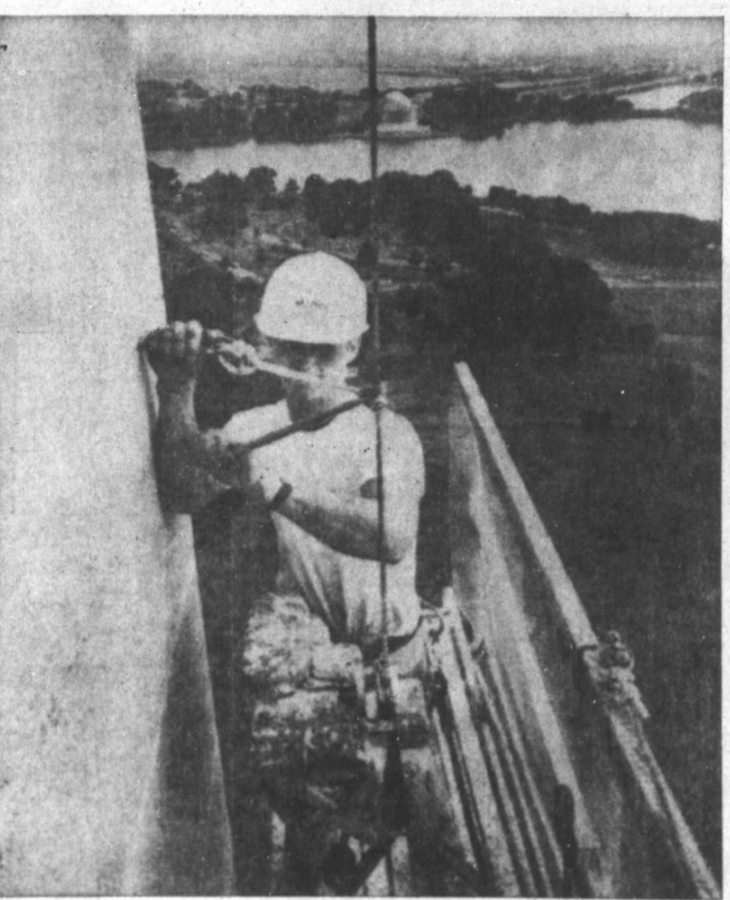
Lofty Labor Bud Tharp secures the cable on his portable scaffold at the 250-foot level on the outside of the Washington Monument. Tharp is foreman of a 10-man crew digging out old mortar between the stones on the monument and replacing it with new concrete. Photographer Dick Darcey of The Washington Post made the trip with Tharp on the scaffold to get this view which dwarfs the autos on the roads below. Washington's Tidal Basin, where the Japanese cherry trees bloom in the spring, and the Thomas Jefferson Memorial are in the distance. (AP WIREPHOTO)
