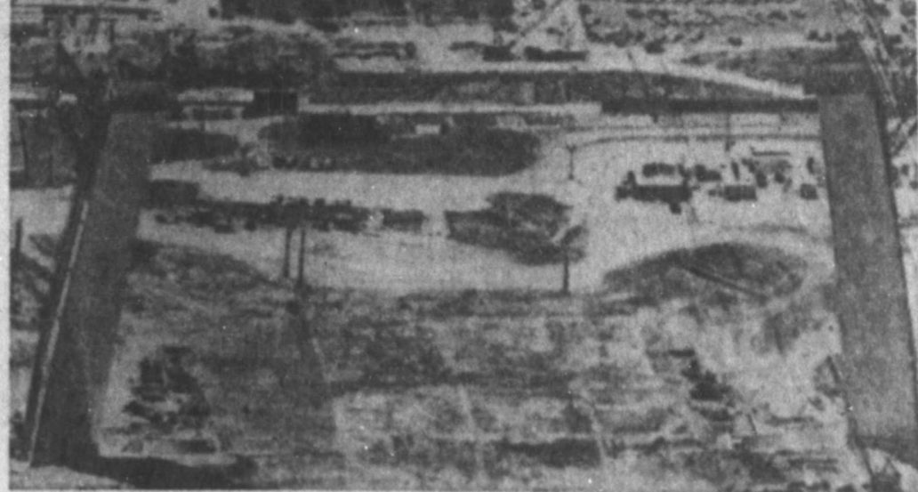
Arch Construction Delayed Work on the Gateway Arch on the St. Louis riverfront has been ordered halted at the 300-foot level for a general appraisal of the project. The north leg (r) presently is 290 feet high and south leg 267 feet high. When completed, the structure will rise 630 feet above the ground. (AP WIREPHOTO)
