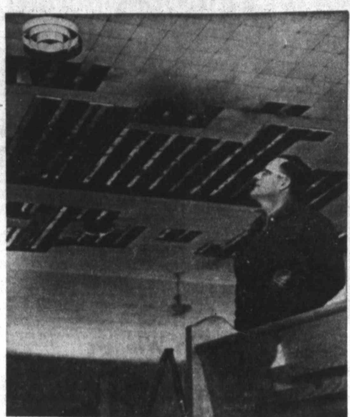
SURVEYS FIRE DAMAGE Pastor Jack Power peers into church attic
