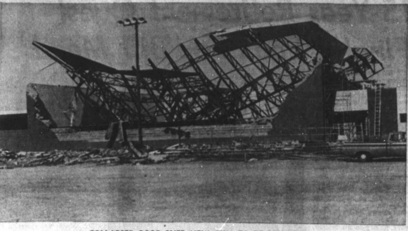
COLLAPSED ROOF OVER NEW GYM TO BE REPLACED Steel roof structure over Klondike gymnasium fell in Sept. 5
