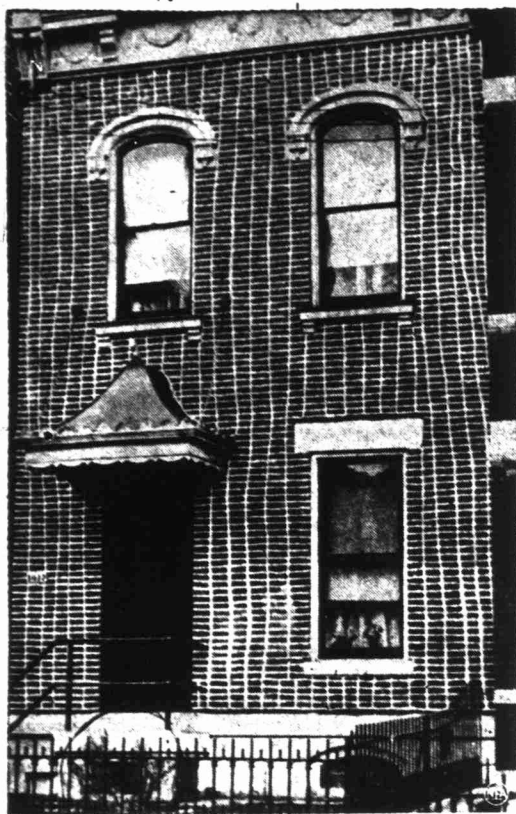
The painter intended to set off the brick front of the home of Samuel Cameron, Cincinnati, Ohio, with neat white stripes. The color was okay, but the lines came out wavy, with the disturbing results above.
