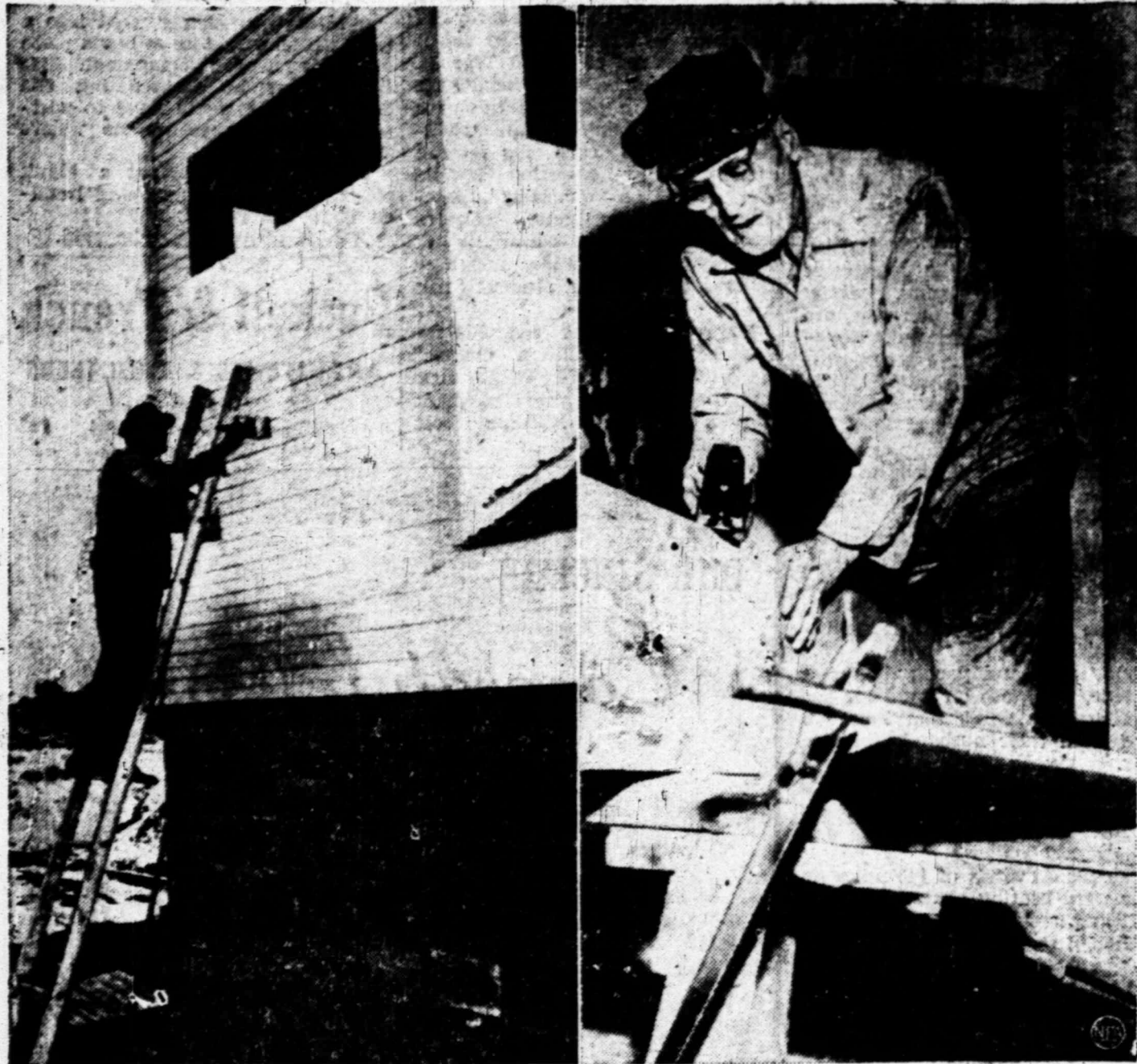
The Rev. D. B. Hampe, 86, of Akron, O., thinks there is religion in hard work as well as preaching. So, donning overalls, he works from dawn to dusk every day to construct his own brick church and a little white frame parsonage. At left, the pastor, a great-grandfather, puts finishing touches to a paint job on his church belfry, and, right, planes a wall board for the parsonage where he and his 83-year-old wife will reside. It's the seventh church Reverend Hampe has started in his more than 50 years of ministry.
