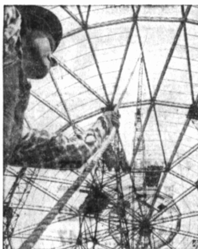
TOP'S ON —Worker guides last truss into place to complete steel framework of dome of the new Houston Stadium. Center is circle at right bottom, 208 feet from ground.
