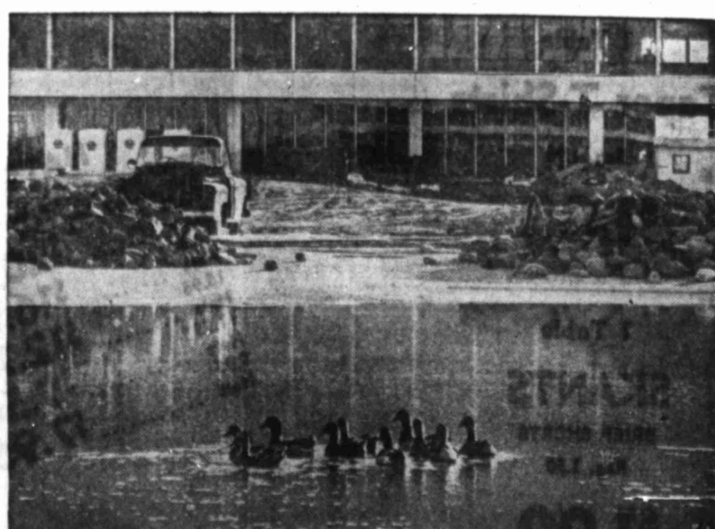
THE FIRST FLIERS —Ten ducks swim in one of the reflection pools behind the nine-story administration building being built for the Manned Spacecraft Center. Construction at the Center, 25 miles southeast of Houston, Texas, is 80 percent complete.
