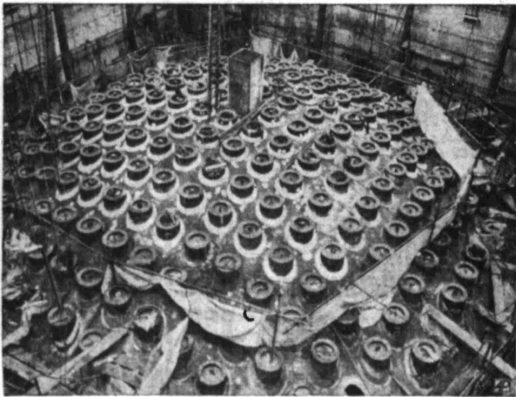
PRESSURE PLUGS —Those wart-like appendages are nozzles welded on top of the No. 2 pressure vessel at the nuclear power station nearing completion at Sizewell, Norfolk, England. Beginning in 1966 the station is expected to produce 580,000,000 watts.
