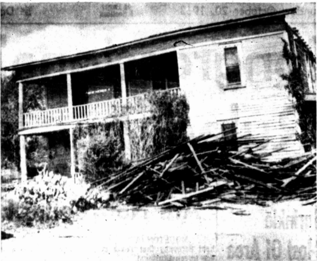
PICTURESQUE OLD LANDMARK TO BE RAZED Residence dates back more than half a century
