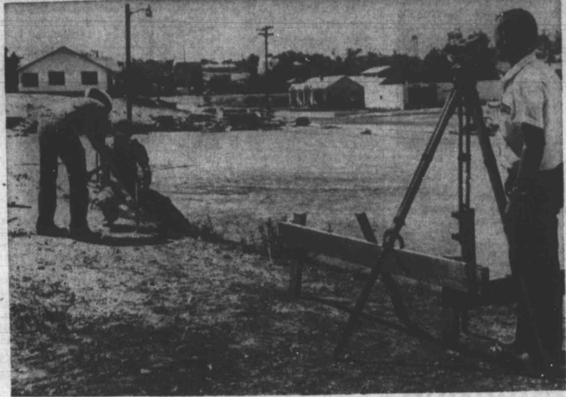
CORNERS PEGGED FOR NEW CLINIC BUILDING K. C. Collier, superintendent, directs operations
