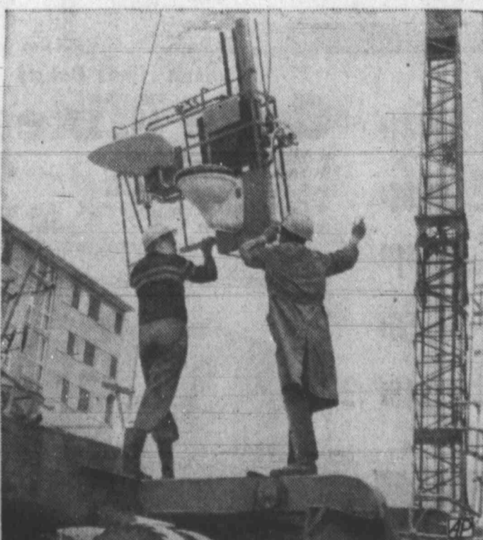
READY TO WORK — A prefabricated bathroom is unloaded in Munich, Germany. Manufacture is geared for speedy installation since labor is expensive and in demand.
