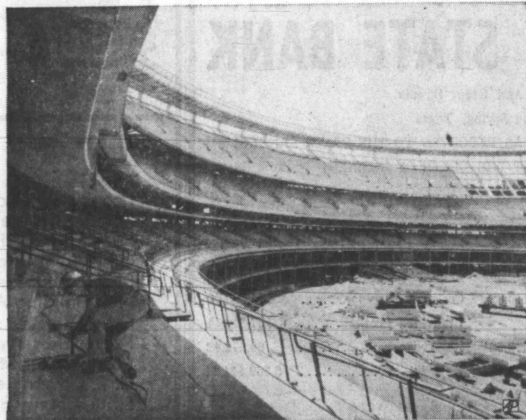
STADIUM TAKES SHAPE —Work continues in the new stadium under construction in Flushing Meadows Park in New York City. The modernistic, pre-cast cement block structure, the future home of the Mets and Jets, is expected to be ready late this year.
