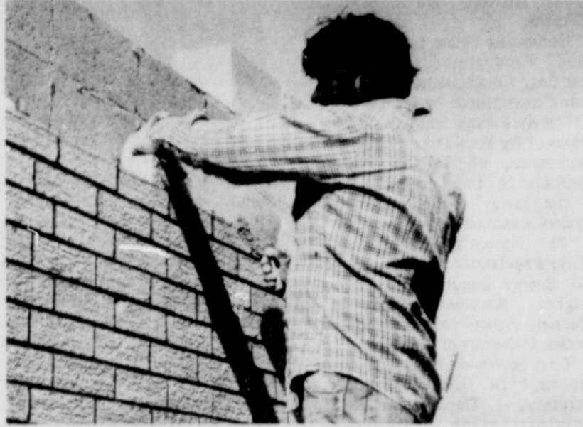
ALLSUP'S WORK.... The construction work continues at the new Allsup's store on East Highway 60. Bricklayer Emello Vuittonet is shown completing a row of bricks. The brickwork was finished this week, and pouring concrete is still underway. Barring delays from the weather, an October 1 opening date is projected for the store.
