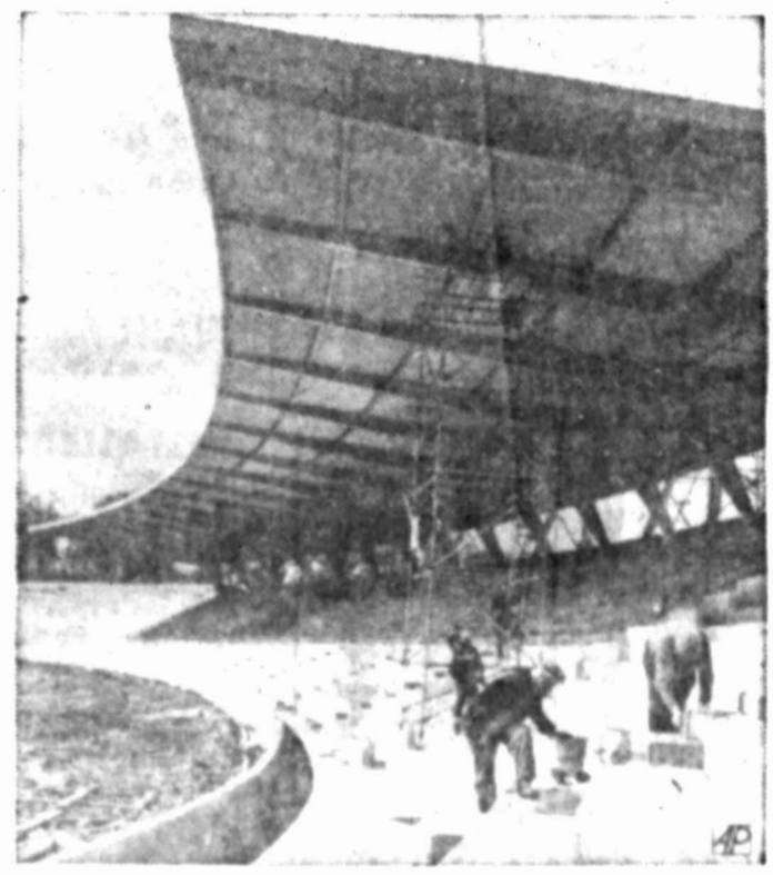
BUILT FOR FUN —Cantilevered roof rises over workers in stadium, part of Crystal Palace Recreation Center, built on site of the old exhibition grounds in London.
