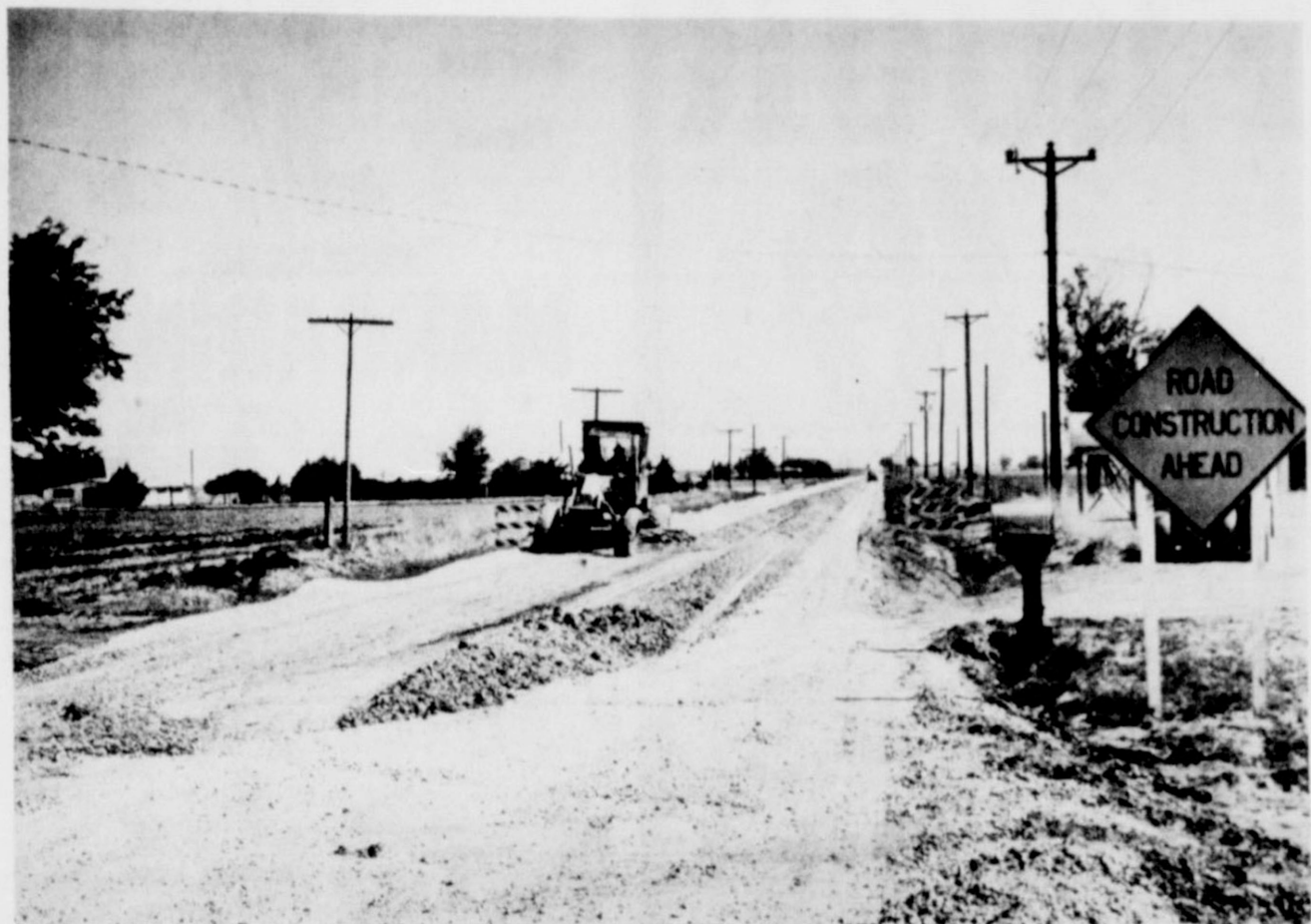
ROAD CONSTRUCTION BEGINS... Work has begun this week on the cemetery road which is in the process of being paved. In the above photo a maintainer is leveling off the road that will be ready for use in a matter of weeks.
