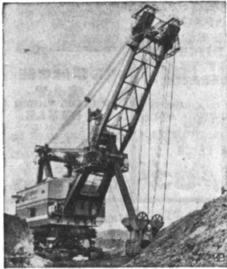
DIGGING AID — Huge stripping shovel stands ready at mine site in western Kentucky after 11 months of assembly. It can uncover 14,000 tons of coal a day.
