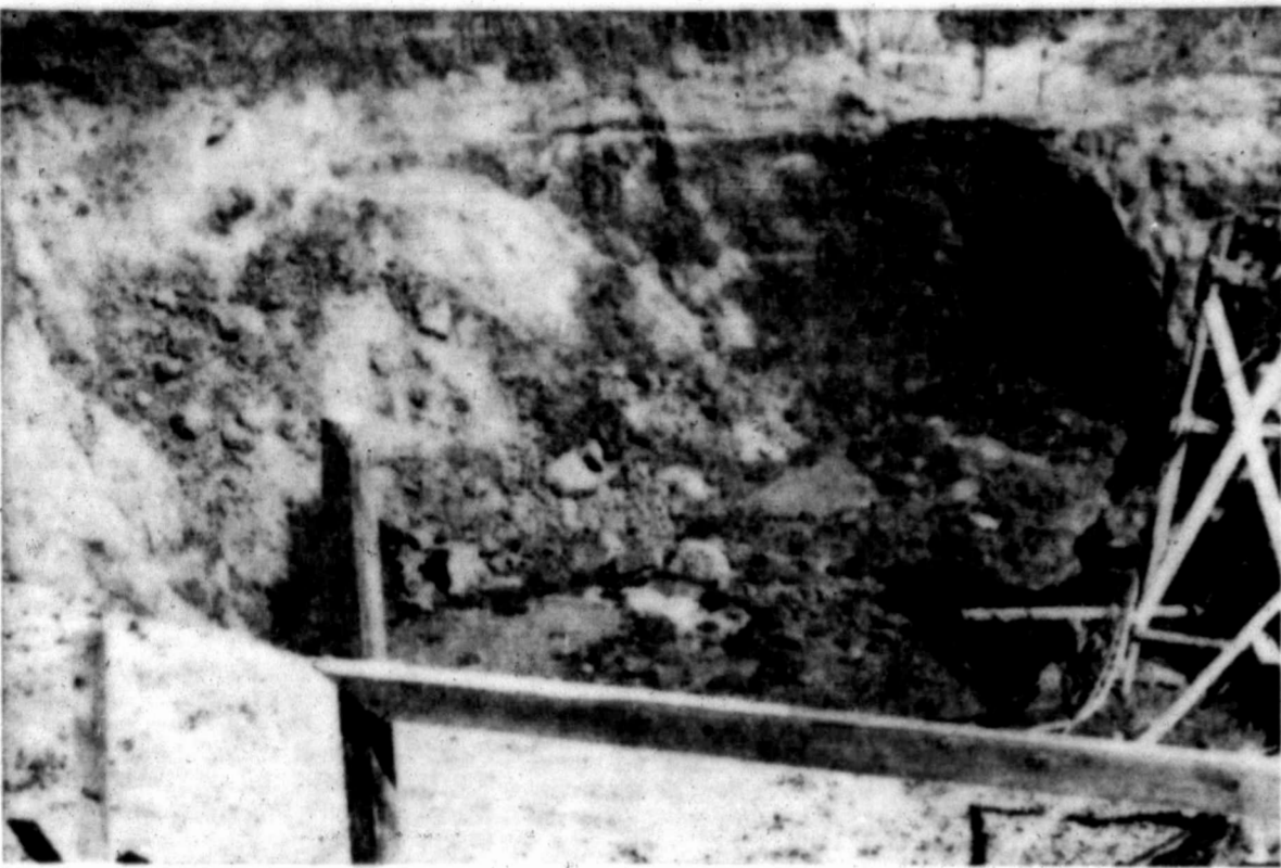
MORE TONS OF DIRT SLOUGH FROM EXCAVATION SIDES Water complicates work for construction crews
