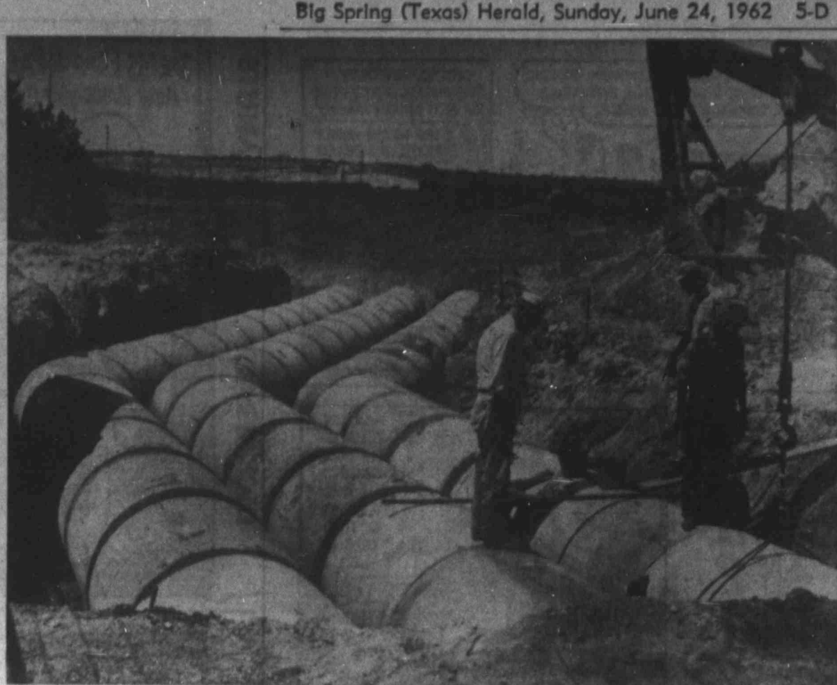
Room For Lots Of Water
