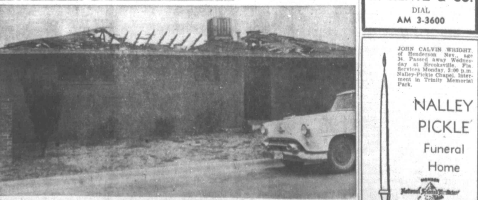
It Took The Roof Off
