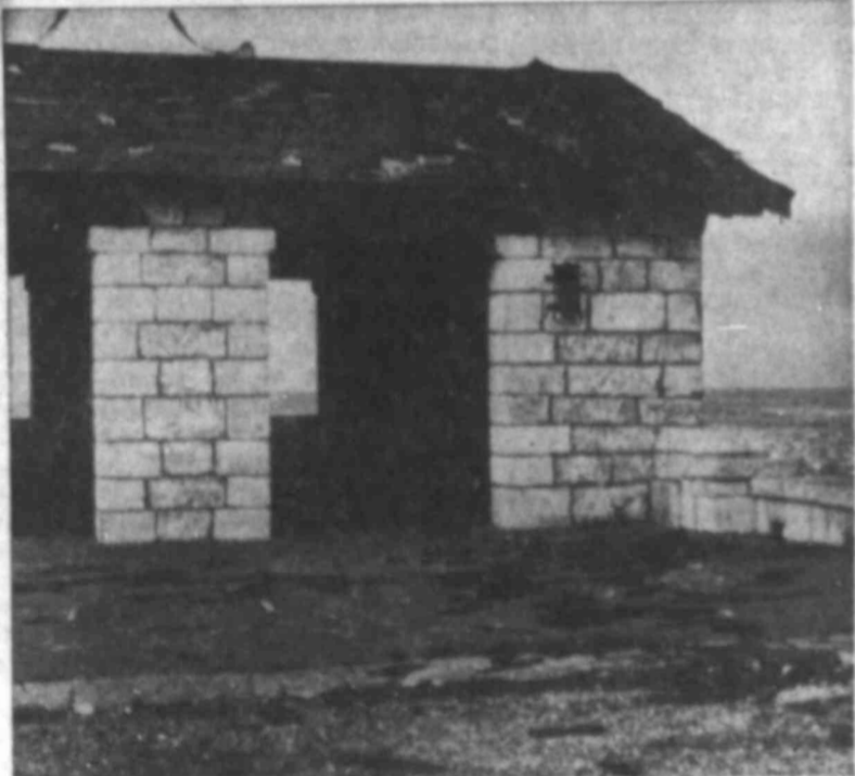
SHINGLES TORN OFF Pavilion being rapidly destroyed
