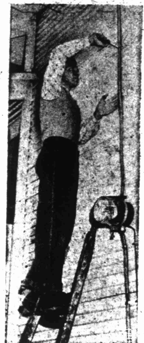
Johnny installed this new three-wire electric service entrance putting new circuits in his home.
