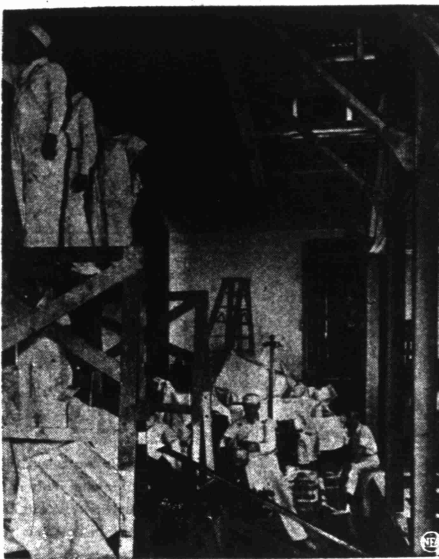
HOUSE CLEANING: Steel beams and squeaky chairs in the midst of which these workmen spruced up the Capitol for 1949 will soon be gone in the first big alteration job since 1859.
