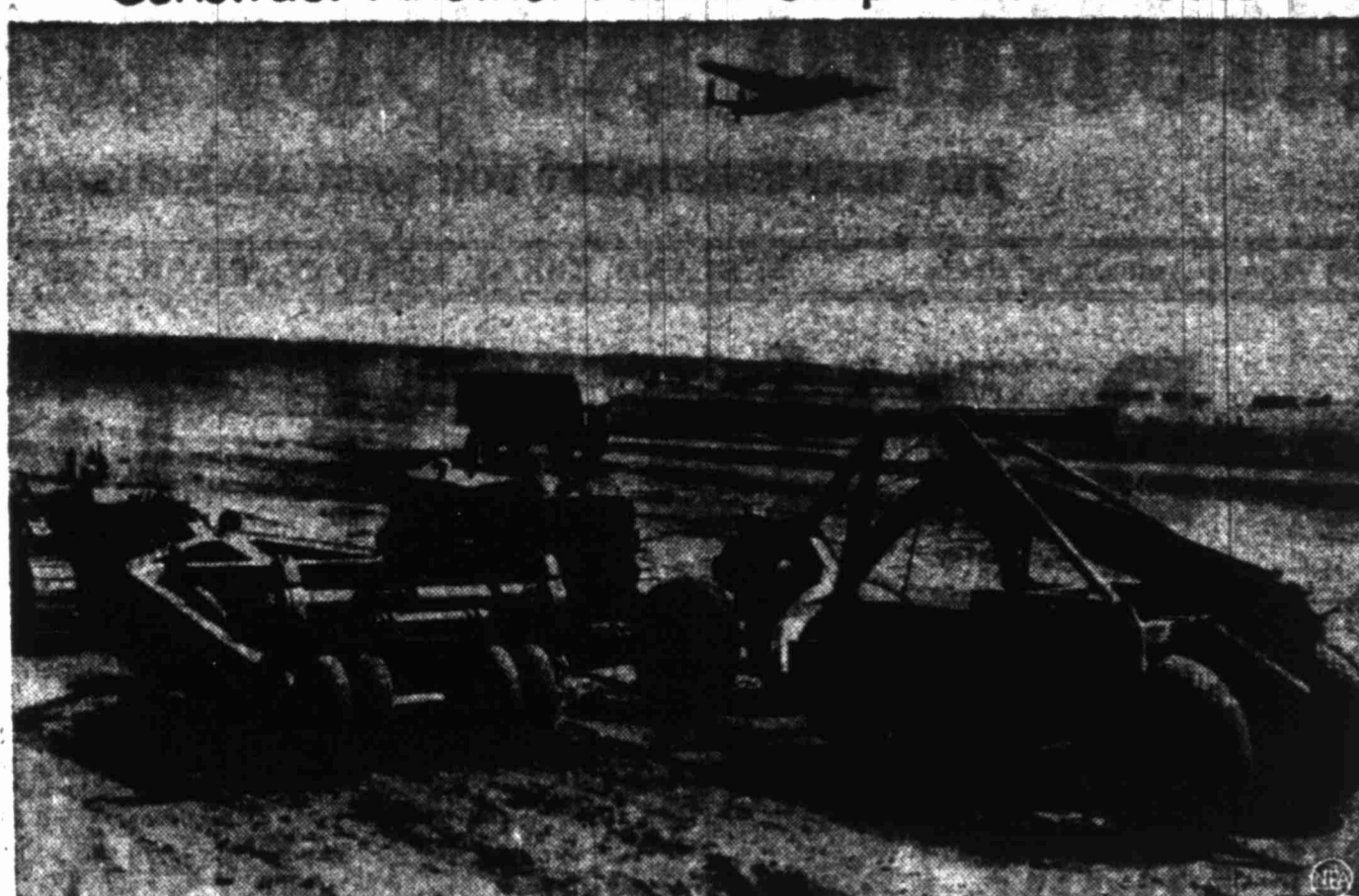
As an airlift plane wings overhead, two bulldozers chug along beginning construction of a new runway at Gatow Airfield in the British sector of Berlin.
