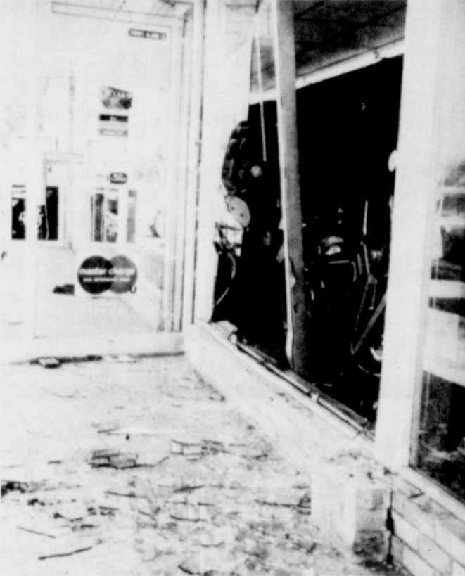
INSPECTING DAMAGE.... Friona City Patrolman, Bob Davis, left and Don Ballew, right, inspect some of the damage inflicted last Thursday afternoon at White Auto Store on West Highway 60. Approximately $700 damage was done to the store when a car driven by Rodolfo Moreno Corella crashed through the large plate glass window in front. Officers said his brakes failed.
