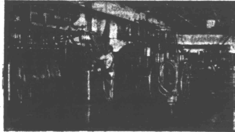
2. Oil pipe lines have worked wonders in all transportation to carry your record demand for oil. This is the interior of Humble Pipe Line Company's pumping station at Comyn. This company operates 8,703 miles of oil and finished products pipe lines in Texas and New Mexico. Though construction of additional pipe lines has been slow because of the high demand for steel for other purposes, the Humble Pipe Line Company has been able to handle the largest volume in its history; during 1947, main trunk lines delivered 253,000,000 barrels of oil.
