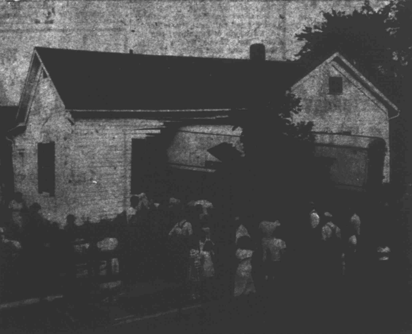
Skidding on a slippery highway, this trailer truck—17 tons of vehicle carrying machinery—careened into the house of Mr. and Mrs. Elton Rasmus, New Beach, O. The truck practically buried itself in the house, and the cab slammed into the bedroom of 11-year-old Billy Rasmus. It just missed his bed, and didn't even wake him up. Driver Lester Snodgrass, of Chicago, escaped with scratches.
