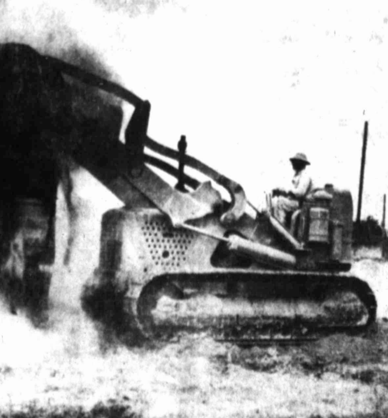
Excavation of the hole for a new three million gallon clear well has begun. The site is between Fifteenth and Sixteenth streets at Virginia. Additional filters with a capacity of 2.25 million gallons a day will also be part of this expansion program, according to Roy Hester, water department foreman. Work should be completed about November.
