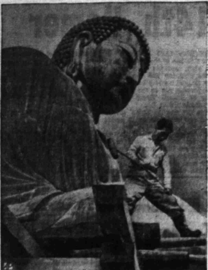
SHORING UP —The base of the Buddha at Kamakura, Japan, is reinforced to make it earthquake proof. The statue was elevated for a steel and concrete foundation.
