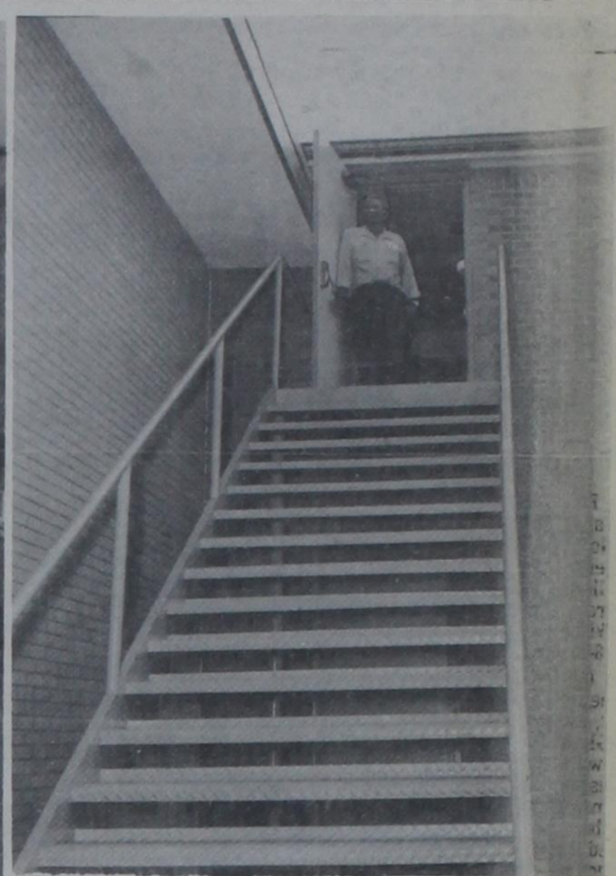
NEW BACK DOOR —Conforming to fire safety standards, the second-floor living quarters in the new city fire station have this "fire escape" back door and steel stairway. "This will probably be the main way we'll come and go," said Fire Marshal Guy Waldrop (in doorway).
