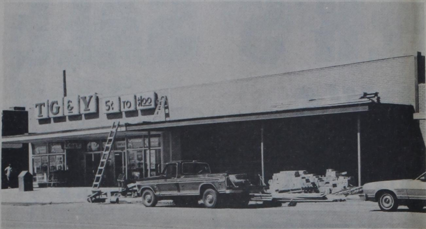
TG&Y EXPANSION PROJECT ON SOUTH BROADWAY ... Workers ready to start on interior now
