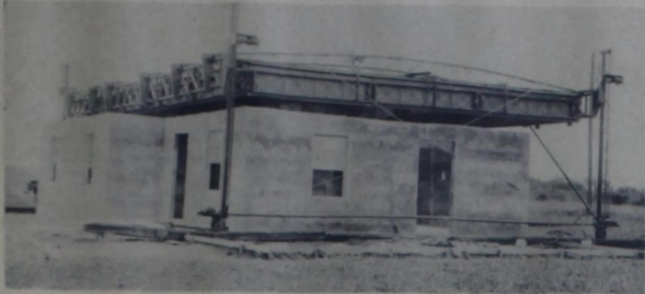
CLIMBING FORM ASSEMBLY COMPLETES WALLS, STARTS MOVING AWAY . . . Prototype concrete home built near Beeville last Thursday
