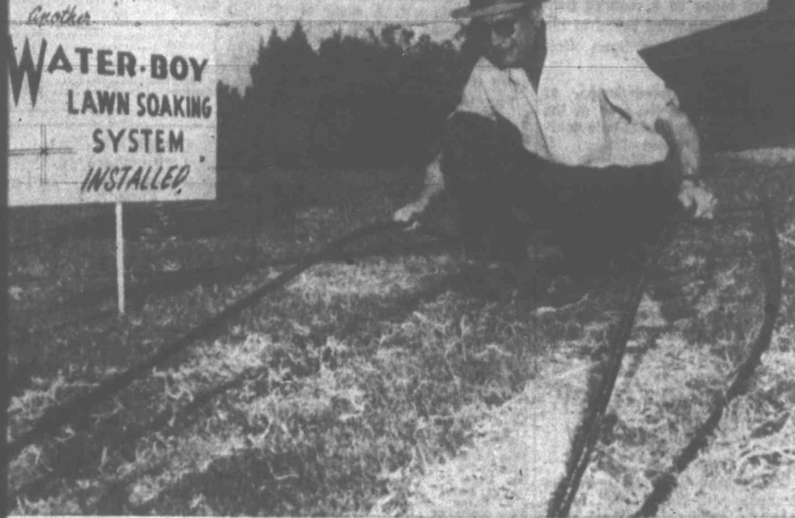
New Water Boy System E. E. Posa displays the polyethylene tubing which became one of the first families in the Big Spring area to install the process at their home at 1600 Park Hill.
