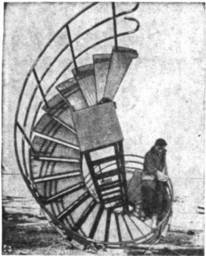
GROUND TEST — Workman negotiates the spiral staircase to be fitted inside the lighthouse being built for the shingle headland into the Channel at Dungeness, Eng.
