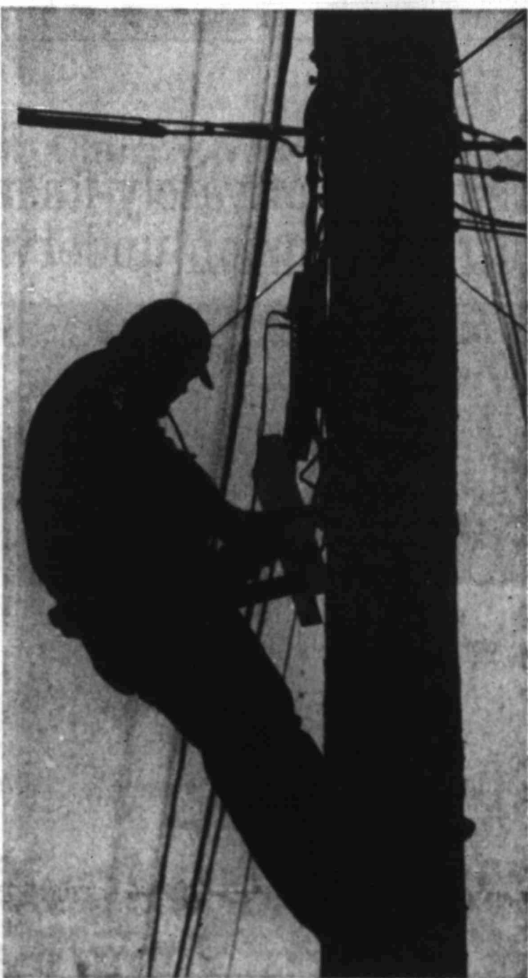
MAN UP A POLE This lineman symbolizes growing demand for utilities
