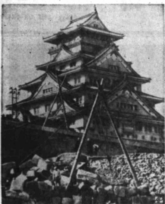
TIME RAVAGE —Workers repair the wall of huge granite stones which fence Osaka Castle, one of Japan's national treasures. Stronghold was built in 1584.
