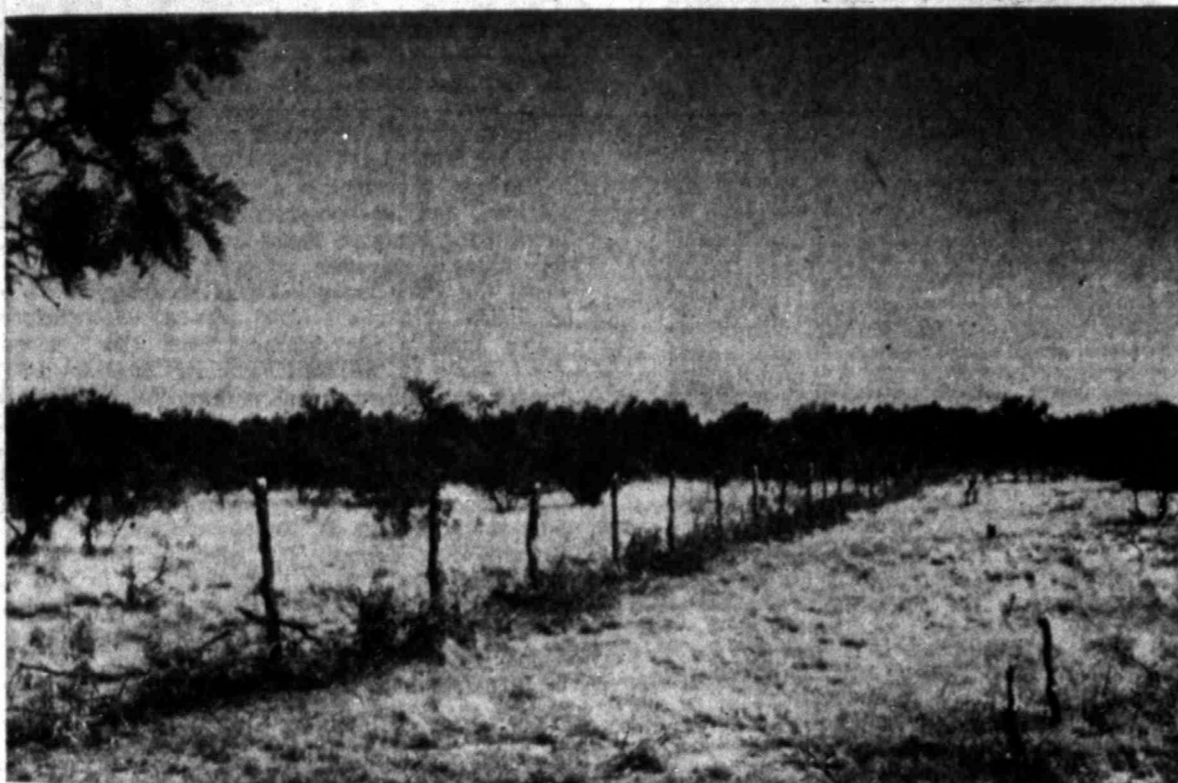
NET WIRE FENCE GOOD TEMPORARY DAM ... Device slows flow of water and spreads precious moisture.
