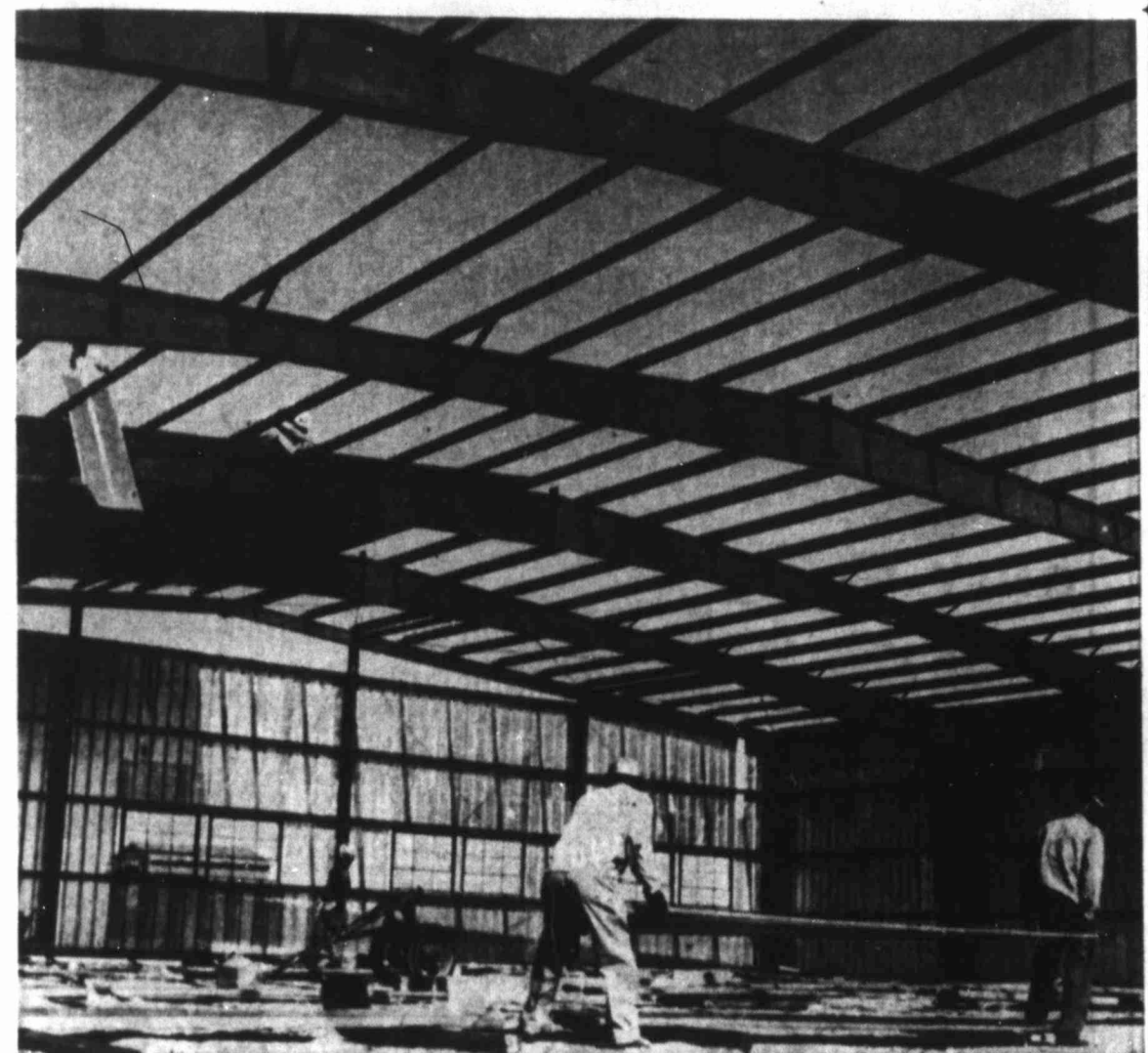
100-FOOT STEEL GIRDELS SPAN COSDEN HANGAR Workmen adding sheathing to new airport structure
