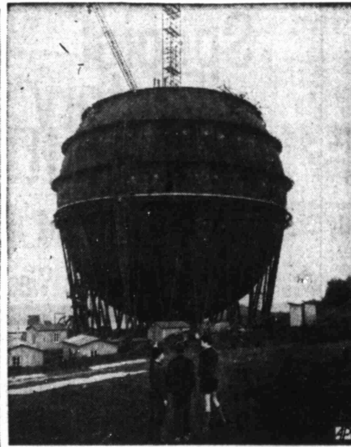
RUHR SIGHT —Youngsters eye giant spherical gas storage tank under construction at Wuppertal, Germany. Steel tank will have capacity of 8,000,000 cubic feet.
