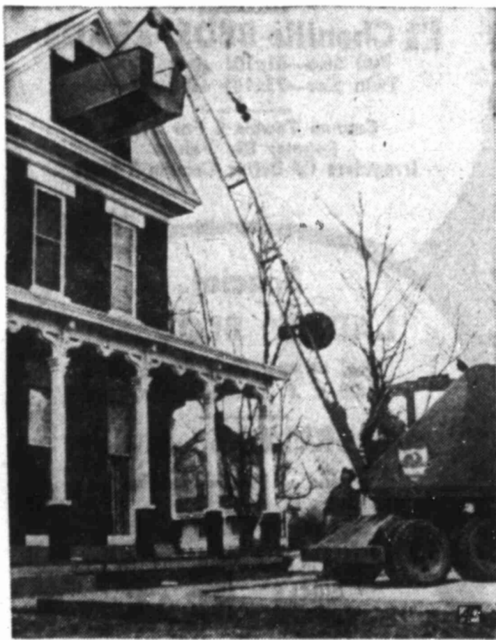
ATTIC LAUNCHING — A do-it-yourselfer had to hire crane to get boat he built out of his attic in Quincy, Ill. Parts of wall and window came out with the boat.
