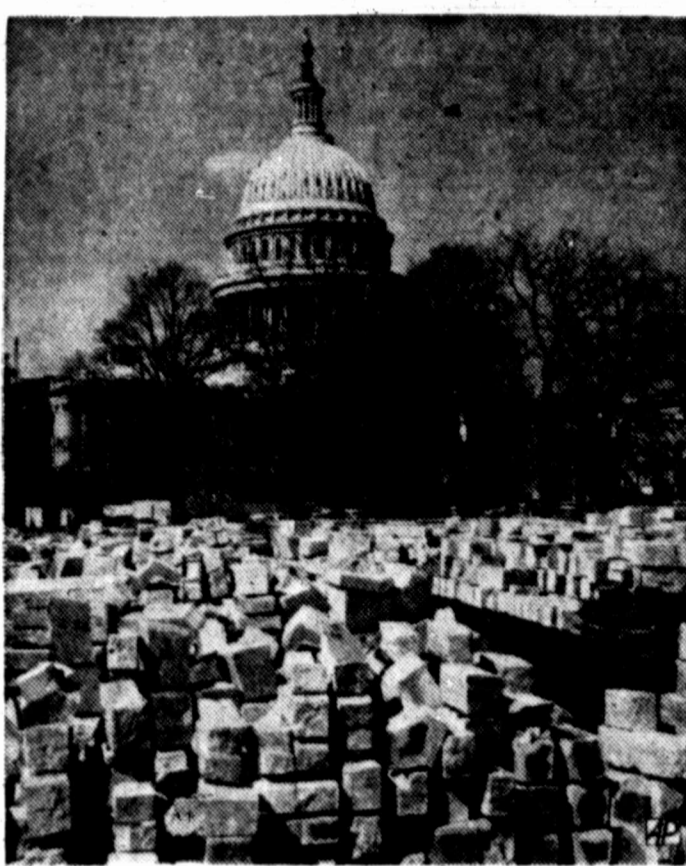
BLOCK CHANGE —These stacked sandstone blocks are part of masonry removed from the Capitol in remodeling project. They'll be replaced by marble blocks.
