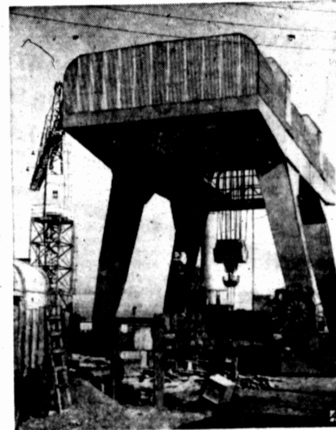
GIANT LIFT —A huge 225-ton crane straddles flood gates of tidal estuary of the Rance river at Saint Malo, France, to lower equipment to harness the tides.
