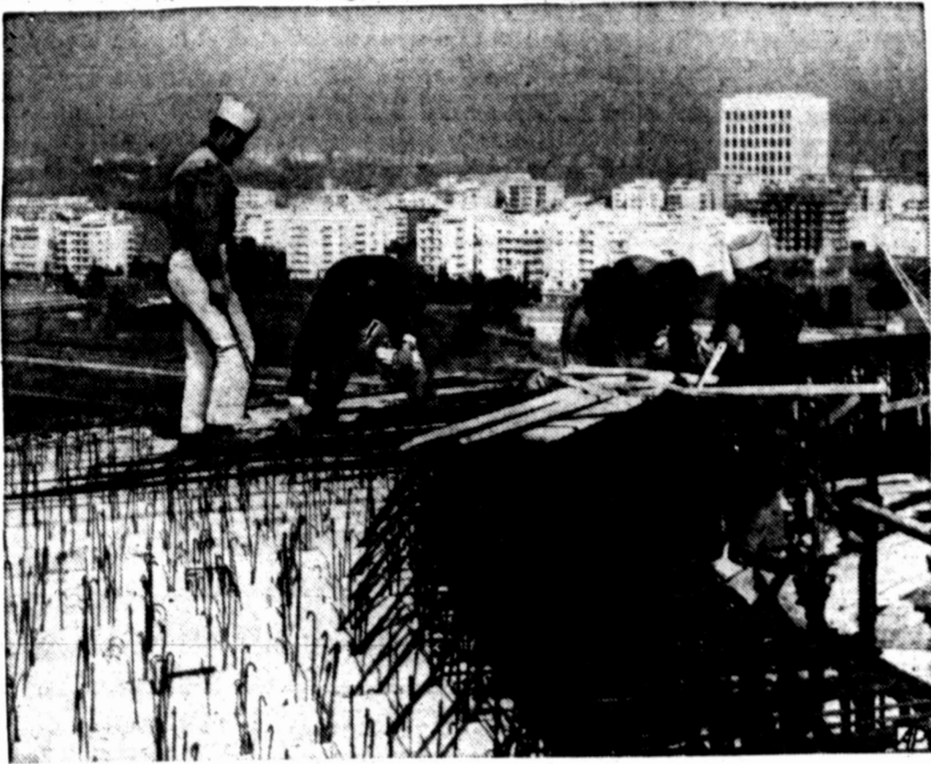
PREP FOR BIG GAMES — Laborers set up concrete reinforcements for arena under construction at Rome's EUR exposition grounds for the 1960 Olympic Games. Arena will be air-conditioned and is to provide facilities for a record entry of athletes.
