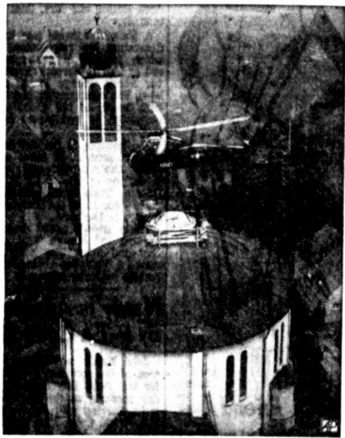
ARMY HELPS CHURCH — U. S. Army helicopter hoists 1,400-pound plastic cupola atop roof of circular-shaped Catholic church at Mussbach, West Germany.
