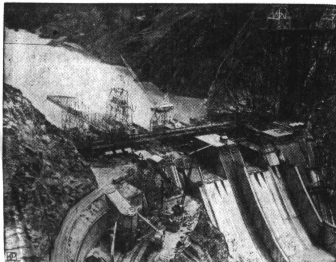
HIGH IN HIMALAYAS — This is the huge Bhakra Dam being built on the Sutlej river north of New Delhi. When completed, the dam and reservoir will supply power and irrigation for an area the size of Belgium in the northern Punjab.
