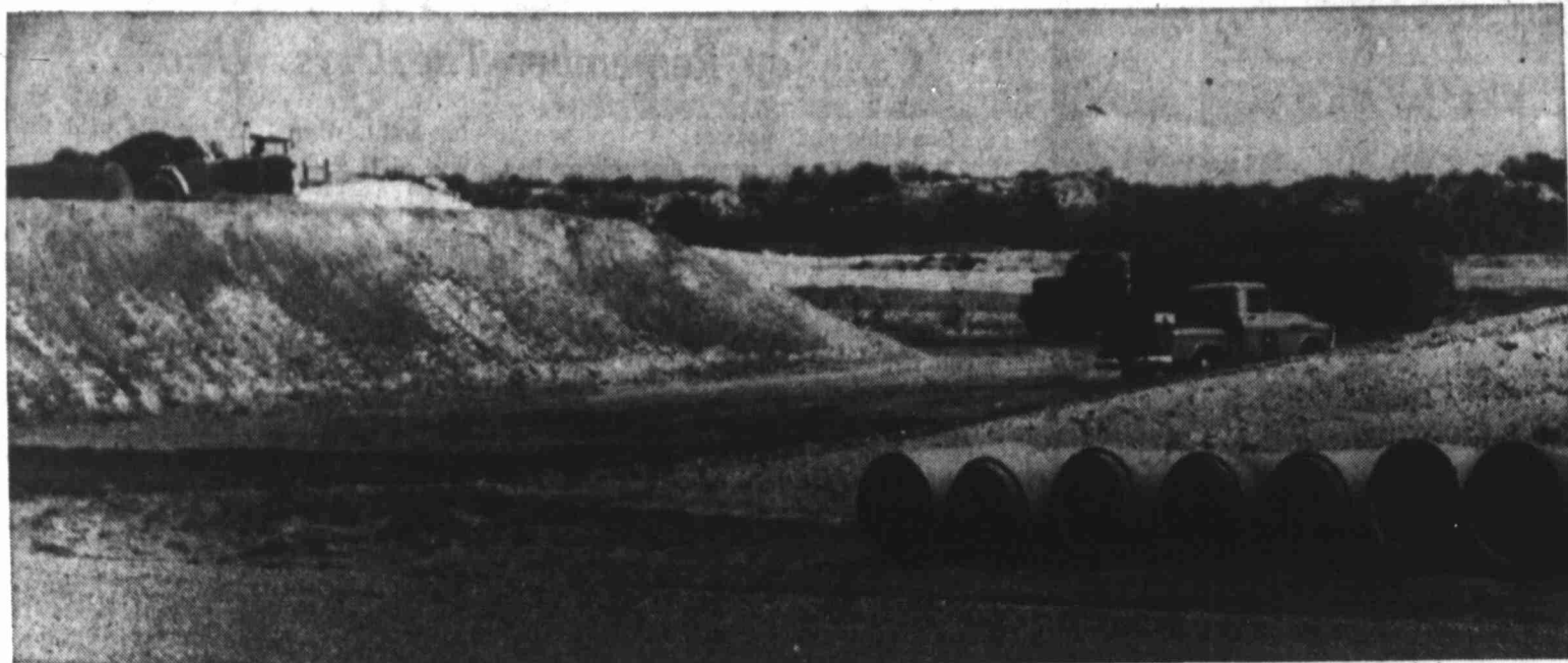
OVERPASS TAKING SHAPE BETWEEN BIG SPRING, REFINERY Eleven such structures being raised in east half of county
