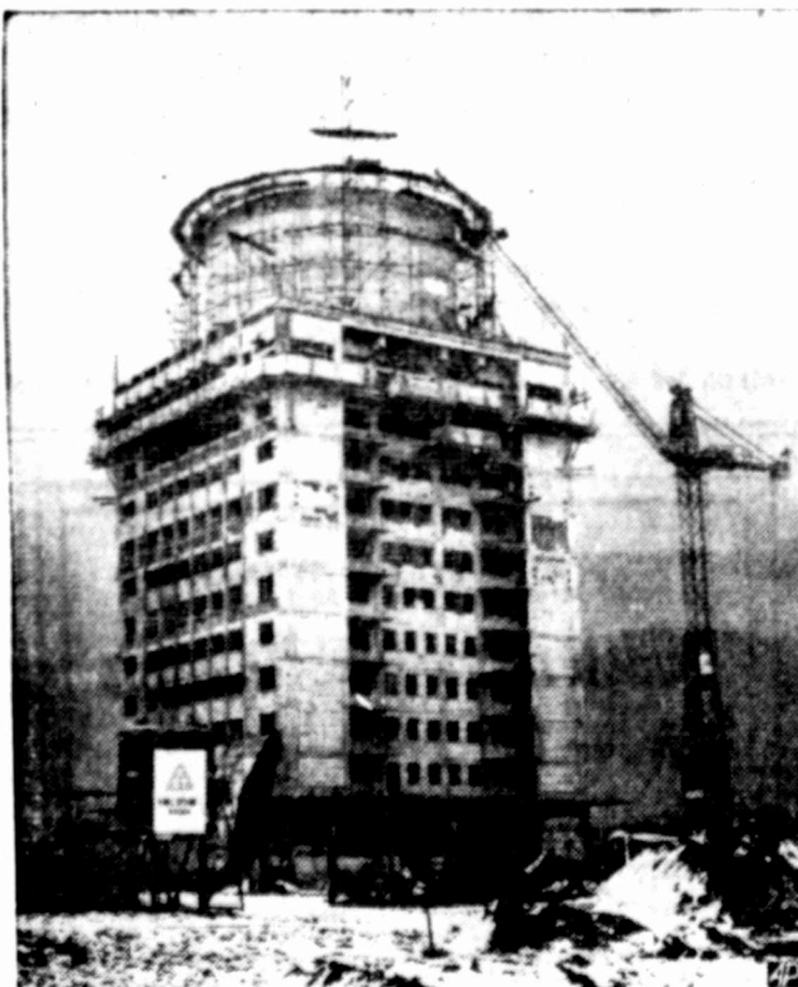
DUAL PURPOSE — Frame of this 12-story apartment house in Velbert, Germany, is built around a water tower. Project disguises tower and conserves valuable ground space.
